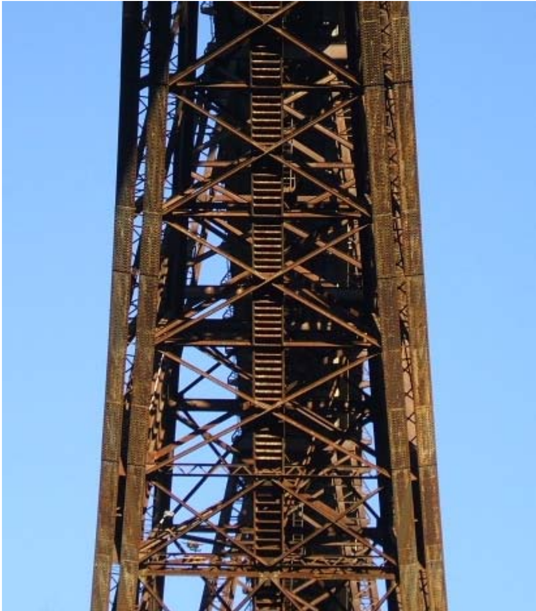
Fig. B7: Prospective view of the arch of the bridge; particular on: the two couples of secondary inclined arches, the transverse brace systems and the boardwalk located into the arch's body.
