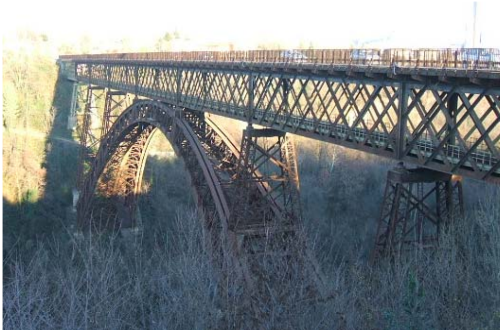
Fig. B1: View of the Paderno d'Adda bridge from the Paderno bank.
