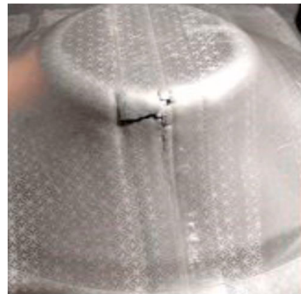
Fig. 6. Welding line failure.
