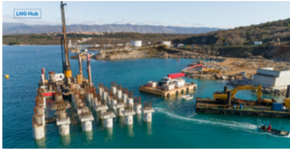
Img. 4: The construction of the docking facility for the LNG-Hrvatska, in 2019-2020. In the background, on the hills, the village of Omissalj (Photo by Balkan Insight).
