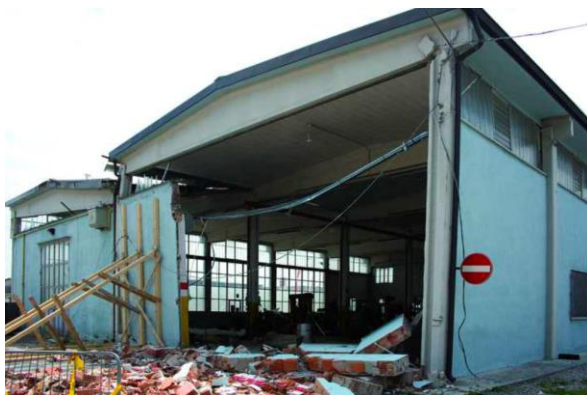
Figure III.22 - The effects of the Emilia-Romagna earthquake on some prefabricated industrial buildings. From [60].
