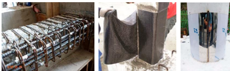
Figure IV.4 - On the left side: beam reinforced with a new RC layer. In the centre: RC column reinforced using CFRP jacketing. On the right side: column reinforced by introducing a steel sheet. From [76].
