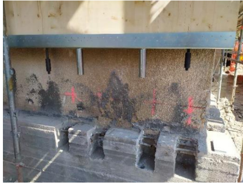
Figure IX.14 - Images of the Structural connections between CLT panels and the foundation at their base. From [247].
