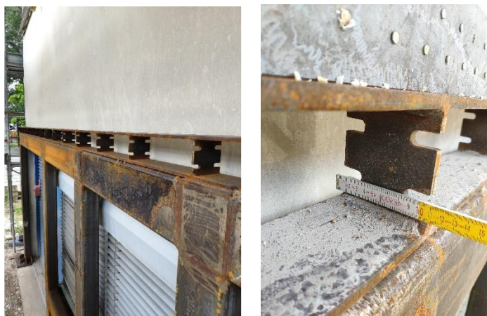
Figure VIII.23 - On the left-side: picture of the AdESA fuses installed along the southern façade. From [15]. On the right-side: detail of the dissipative connection. Picture shot by the author.
