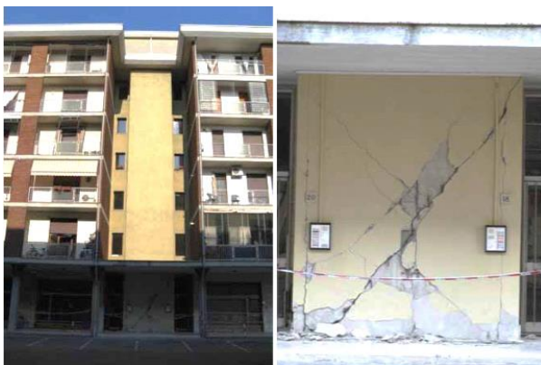
Figure III.18 - Damage at the base of the staircase wall of an RC building caused by the 2012 Emilia, Italy, earthquake. From [44].
