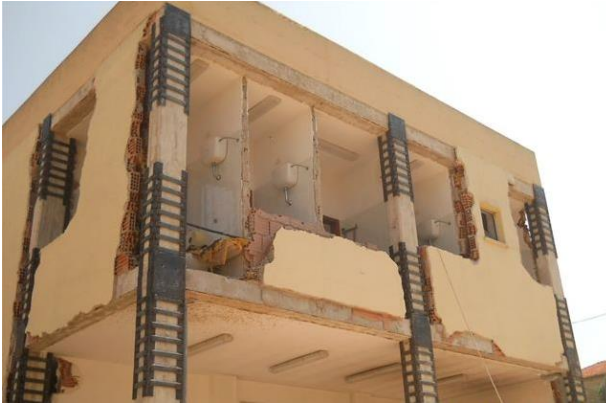
Figure II.10 - Partial finishing and non-structural elements demolition for an intervention of local strengthening of the columns. From [9].
