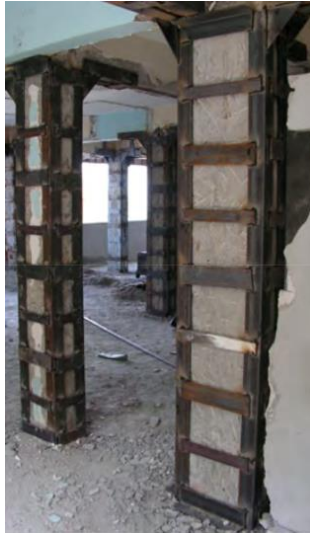
Figure IV.3 - Intervention of local strengthening of the columns requiring partial completion and demolition of non-structural elements and finishes. From [70].
