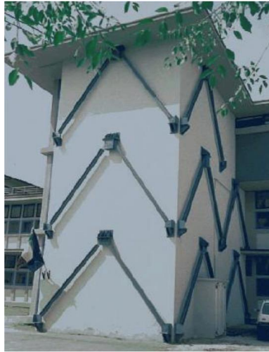
Figure IV.11 - example of retrofitted viscoelastic dampers in bracing configuration. From [93].
