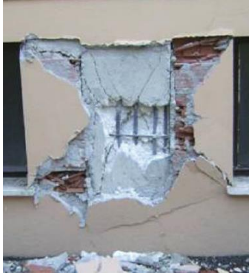
Figure III.15 - Following the L'Aquila earthquake, a partial infill of the frame caused a typical brittle shear failure of squat columns. From [46].
