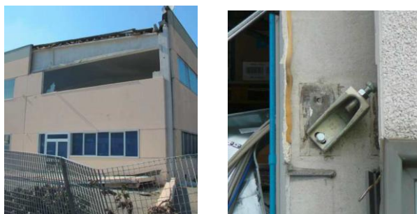
Figure III.21 - Collapse of the horizontal closing panel and its structural connection. Form [56].
