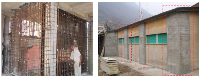
Figure IV.5 - On the left side: construction of new earthquake-resistant shear walls between frame bays. From [81]. On the right side: construction of new external RC shear walls, adjacent to the pre-existence. From [79].
