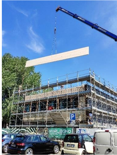
Figure IV.35 - picture of the installation of the structural layer in cross laminated timber panels, shot by the author.
