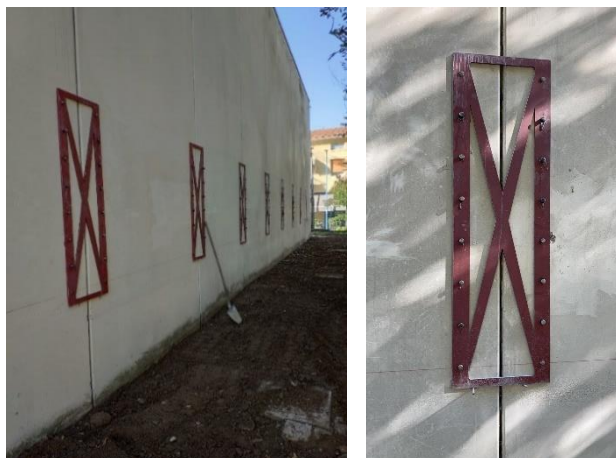
Figure VIII.26 - pictures of the mechanical coupling elements installed between the adjacent RC cladding panels. From [15].
