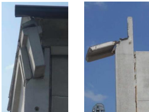
Figure III.20 - Examples of damage and collapse of the reinforced concrete precast joint having the task of providing stability to the roof beam. From [56].
