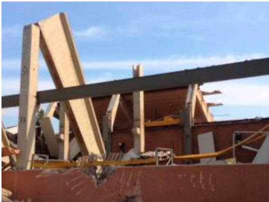
Figure III.24 - Example of the collapse of the roof due to loss of support of its elements. From [56].
