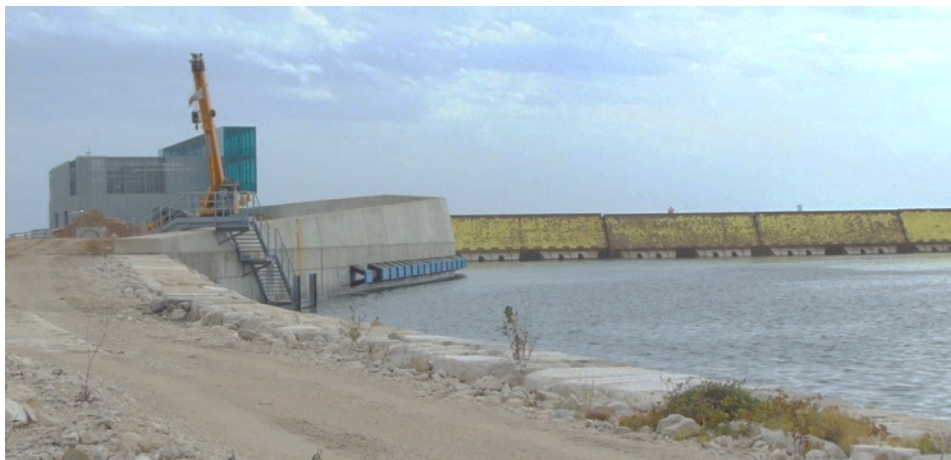
Figure 5 – 3rd October 2020: the MOSE in a raised and working position (author’s photo).
