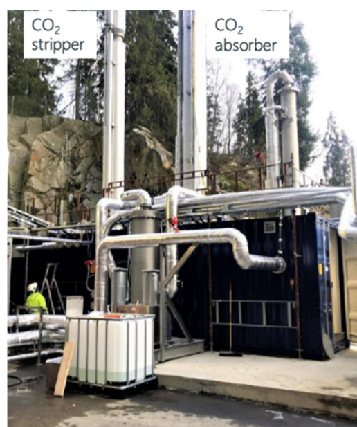
Figure 7. The Klemetsrud WtE + CCS pilot plant (Norway).
