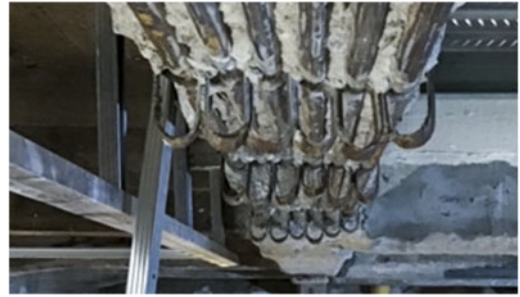
Figure 13. Reinforcements of the perimeter beam after the removal of the damaged concrete cover.
