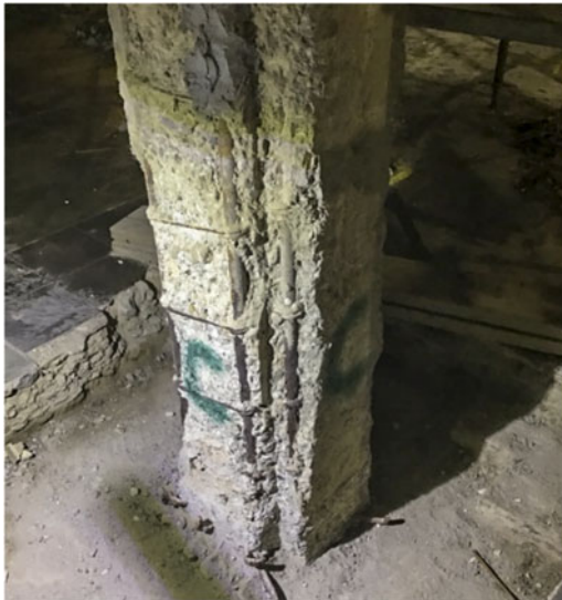
Figure 12. Reinforcements at the base of the pillar after the removal of the damaged concrete cover.
