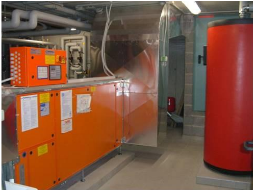
Figure 0-6: The main air-handling unit in the cellar.
