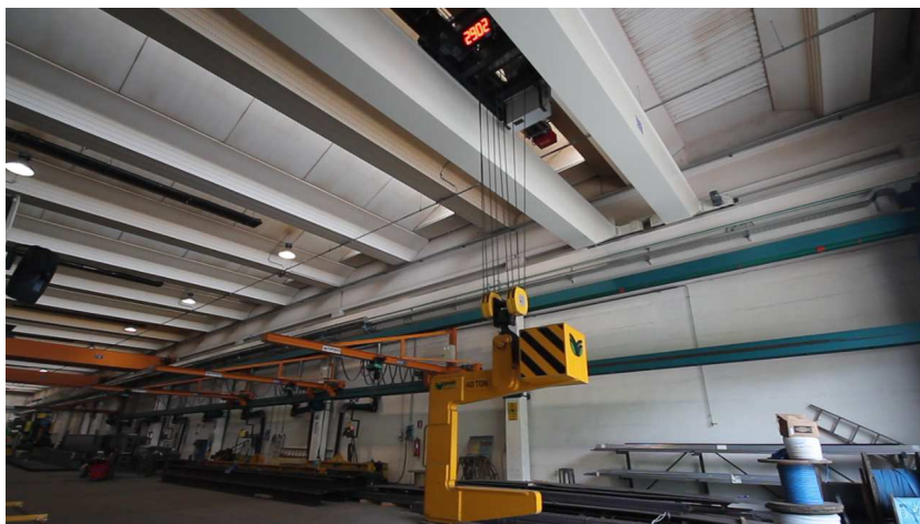
Figure 3.22: The real bridge crane with the C-shape load of 3000 kg connected.
