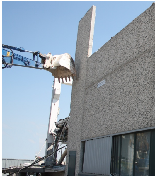
Fig. 1 Horizontal cladding failure after a seismic event
