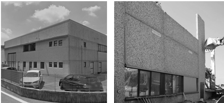
Figure 3.7 Examples of precast industrial buildings with horizontal precast cladding panels. Undamaged panels (left); damaged panels after Emilia earthquake (right).
