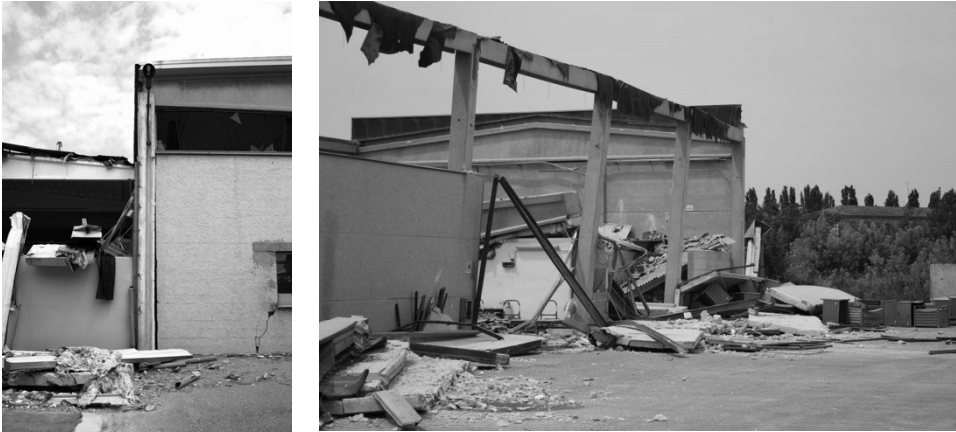
Figure 3.6 Permanent loss of verticality: the presence of a gap in the lower side between the column and the external infills blocks can be observed (left); permanent rigid rotation of the columns in the isolated cup foundations (right).
