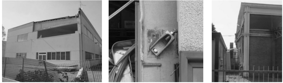
Figure 3.2 Failure of the support of the cladding panel with consequent fall of the panel itself (left and middle); out-of-plane overturning of the masonry infill in a single-storey industrial building (right).
