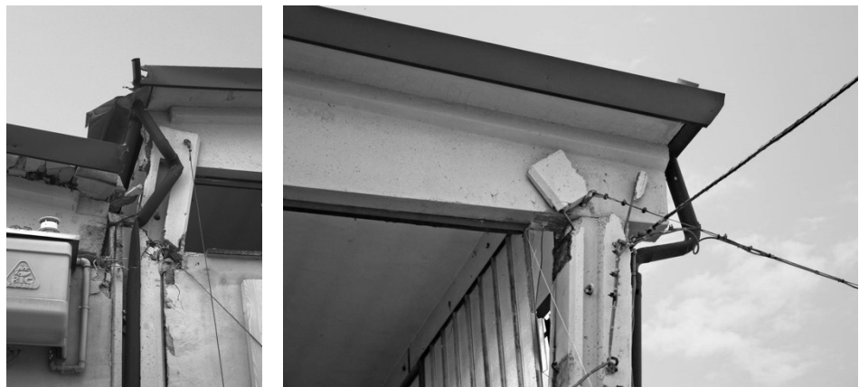
Figure 3.3 Failure of the column due to the presence of infill panels and strip windows (left); failure of the fork at the top of the column due to the out-of-plane stress of the beam (right).
