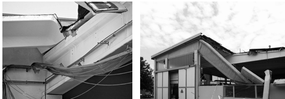
Figure 3.1 Fall of roof elements (left) and fall of I-shaped beams due to loss of support (right). The lack of support at the end of the beam led to a changing of the real static scheme and the beam is collapsed since it has not been designed for the new constraint configuration.
