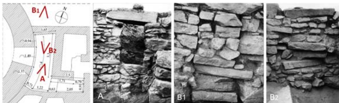
FIG. 16 – VIEWS OF THE TRANSVERSE WALLS OF THE ADJACENT ROOMS ± AND ¥: NO BUTTRESS ACTION IS PROVIDED BY THESE WALLS TO THE CHAMBER RING MASONRY GIVEN THE LACK OF MUTUAL INTERLOCKING AND THE SIGNIFICANT WEAKENING INTRODUCED BY SEVERAL OPENING (ONE HAS BEEN CLOSED IN A SECOND TIME – B IN THE FIGURE).
