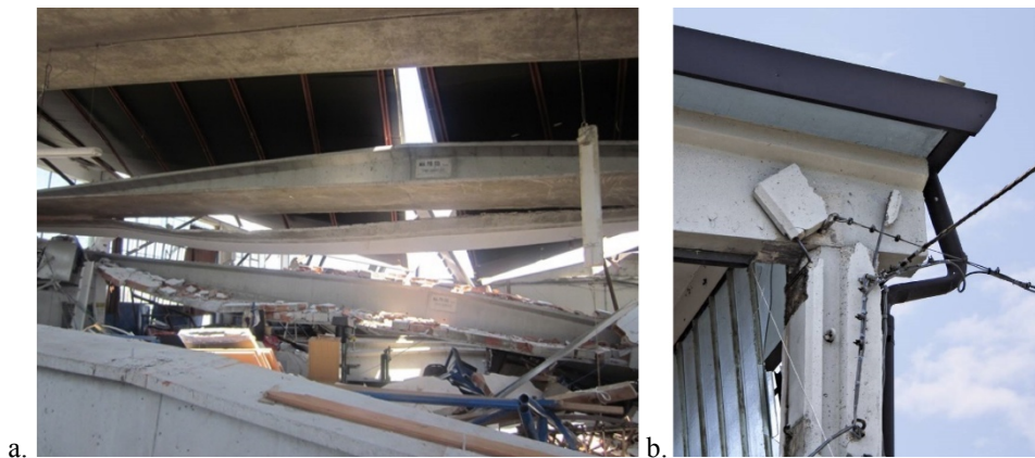
Fig. 1 (a) Damage caused by the collapse of the roof in a RC precast industrial building in Emilia, 2012 (b) failure of the fork at the top of the column due of the out-of-plane stress of the beam.
