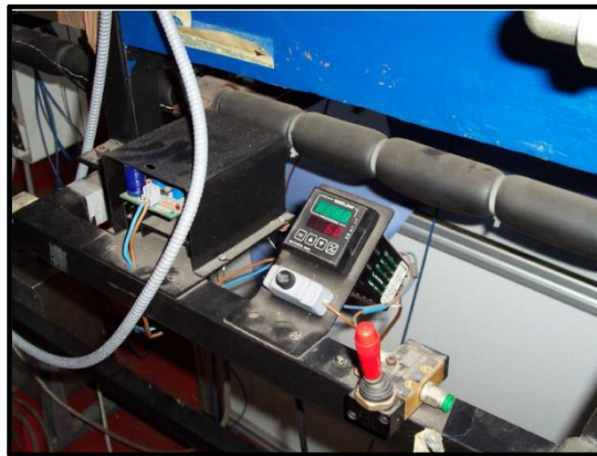
Figure 6.4 : secondary flow pipe with insulated heater and regulation system.
