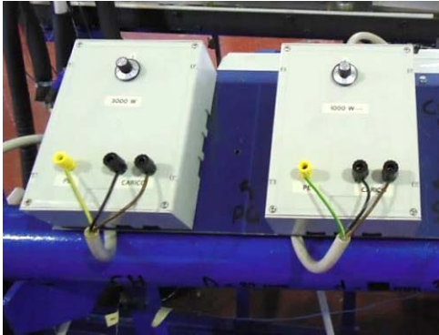
Fig. 3.25- Rheostats using for regulating the power of the electrical heaters
