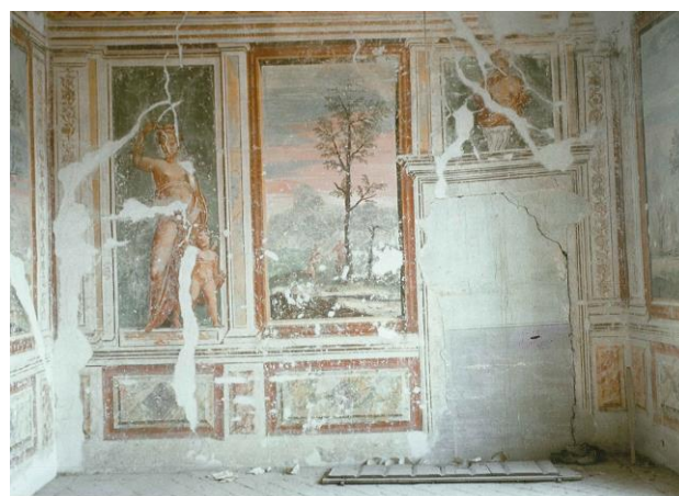
Figure 11: Crack pattern, room 28, 1990 (Private archive Federico Merli).
