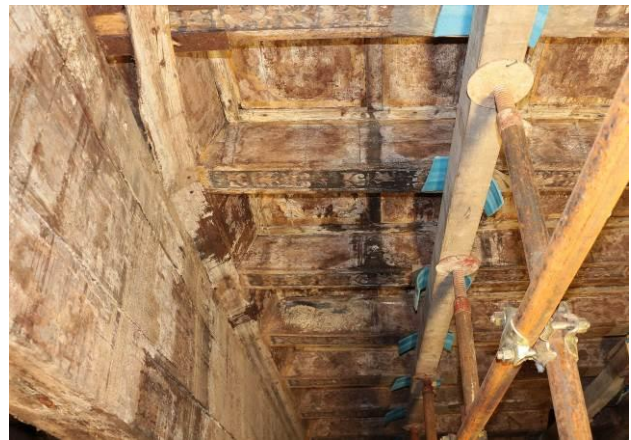
Figure 14: Wood decay, main hall.
