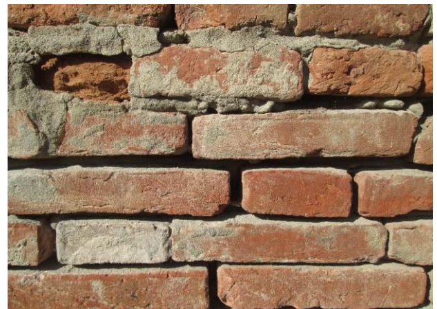
Figure 7: Loss of the mortar.
