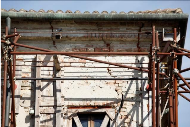
Figure 12: Cracks due to the outward thrust exerted by the roof.
