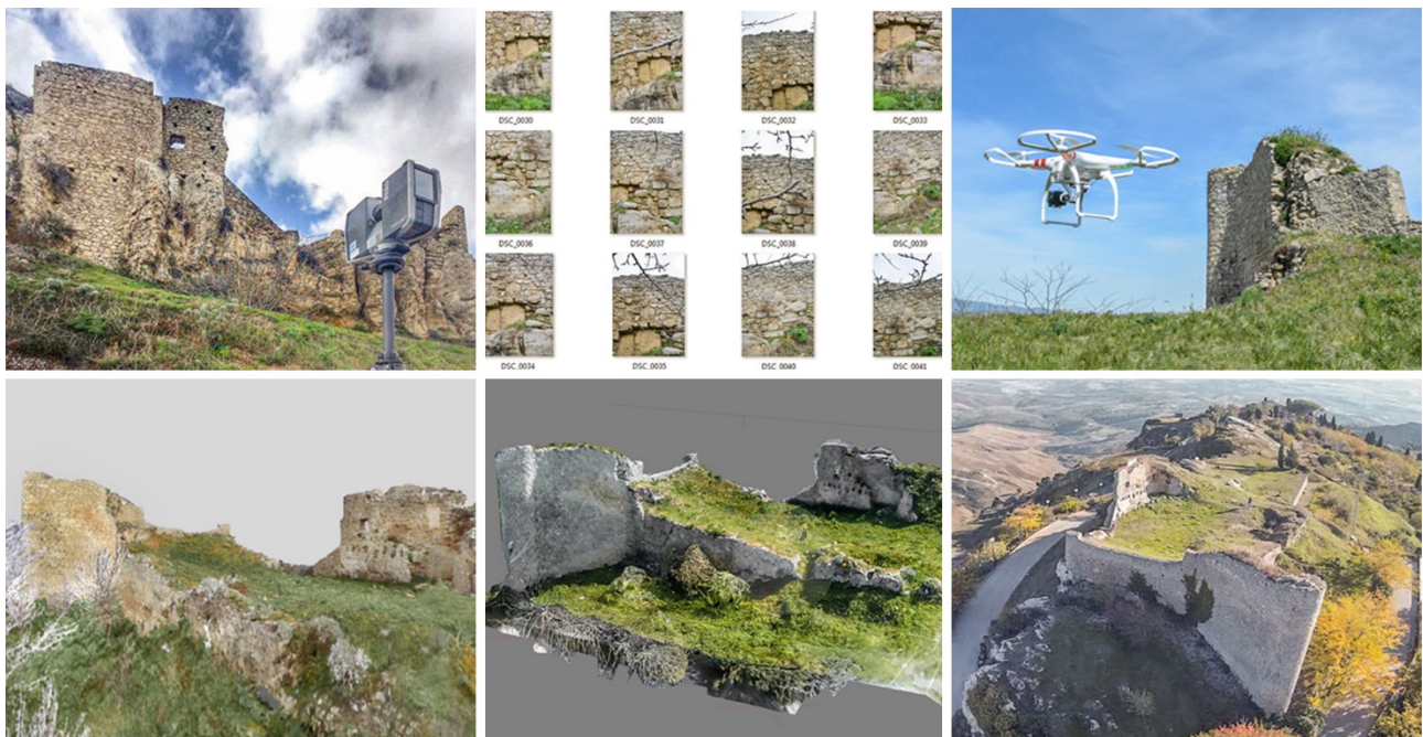
Figure 3. The integrated survey: 3D laser scanning and digital terrestrial and UAV photogrammetry.
