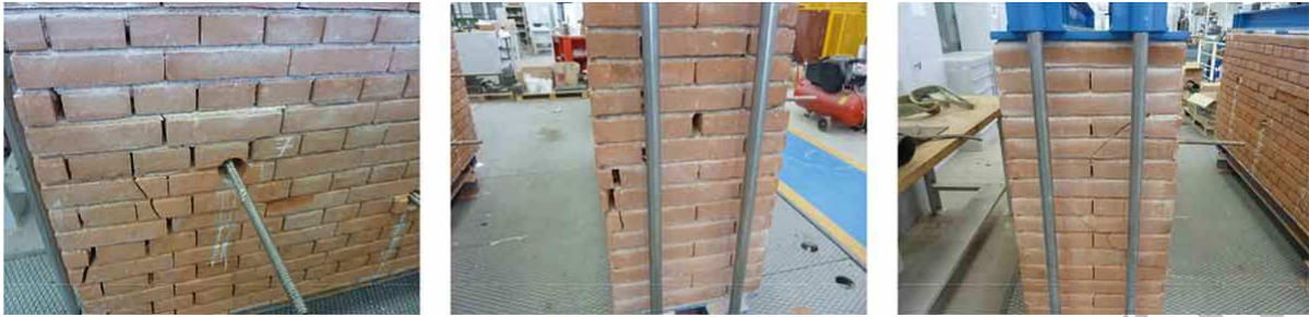
Fig. 17: Failure mechanisms observed in wall I and H after the tests
