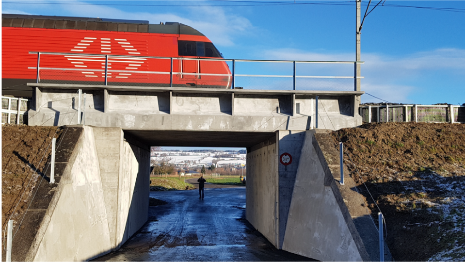
Figure 6.1: View of SU Unterwalden railway bridge (district of Sursee, canton of Lucerne, Switzerland).
