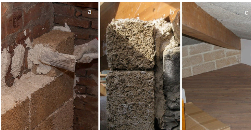
Fig. 1. Details of non-load-bearing walls made of hempcrete blocks: (a) wall erection; (b) side view; (c) front view.
