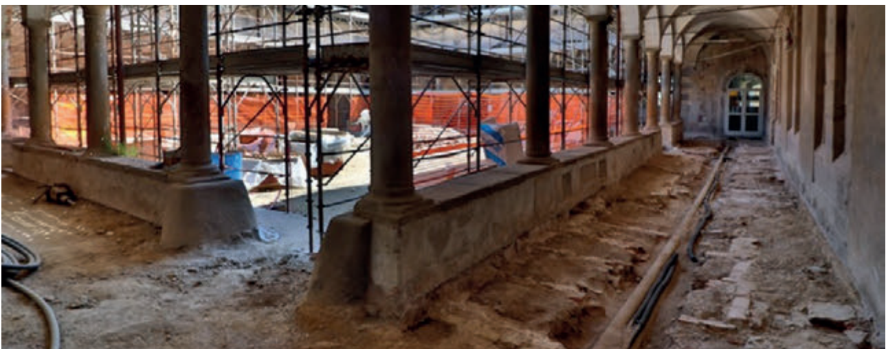
Figure 3. The building site of the small cloister with the tombs and the fragments of epigraphs (©Colleoni, May 2021)
