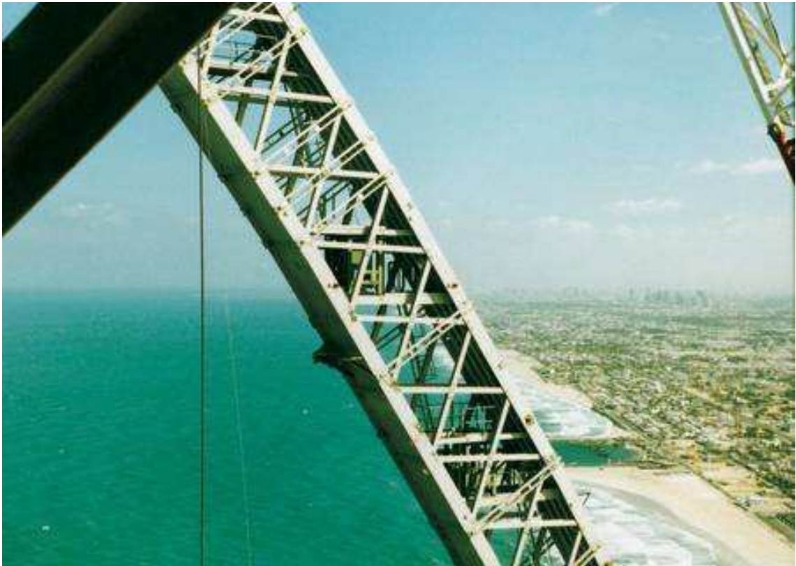
Figure 2.2: TMD placed into the steel arms of the Burj Al Arab hotel in Dubai, UAE, 1999 (Source: Internet, http://www.gerbusa.com ).
