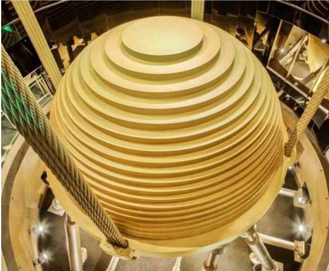
Figure 2.3: The 660 t Tuned Mass Damper placed between the 87th and the 92th floor of the Taipei 101 skyscraper, Taipei, Taiwan, 2003 (Source: Internet, https://buildcivil.wordpress.com ).
