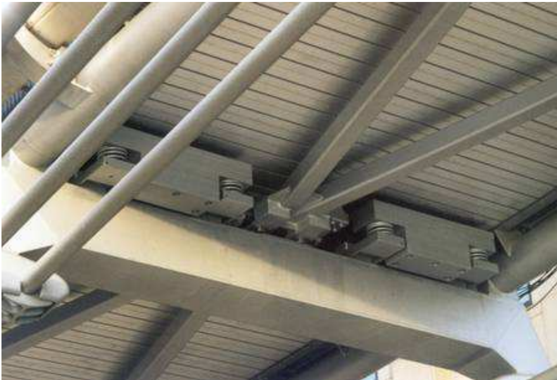
Figure 2.1: Vertical TMDs installed under the footpath of the Millennium Bridge, London, UK, 2001 (Source: Internet, http://www.gerbusa.com ).
