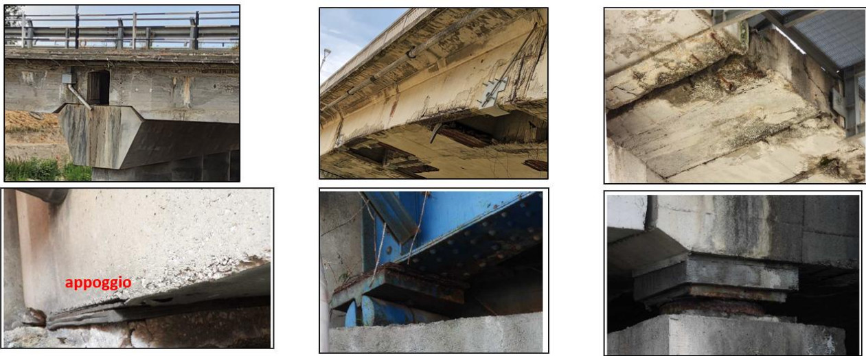
Figure 59: Example of degrading on bridges.
