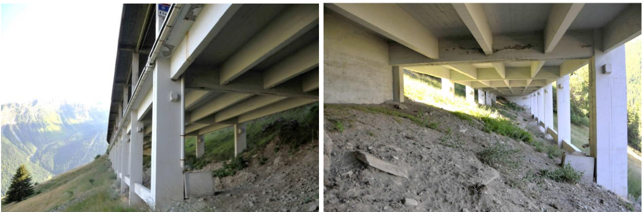
Figure 53: Chantel 2 Viaduct, original design of deck section and nowadays photo of the structure.
