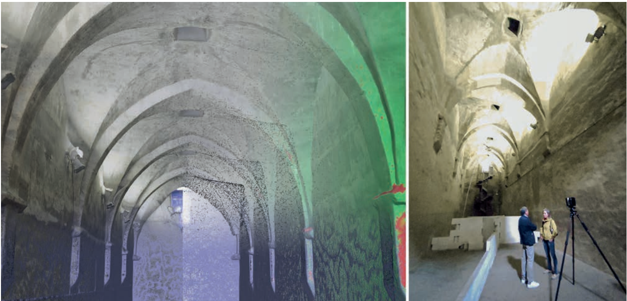
Figure 2. Internal area of Fontanone Visconteo : 3D photogrammetric models mix (overlap between point cloud, mesh texture and confidence indication).
