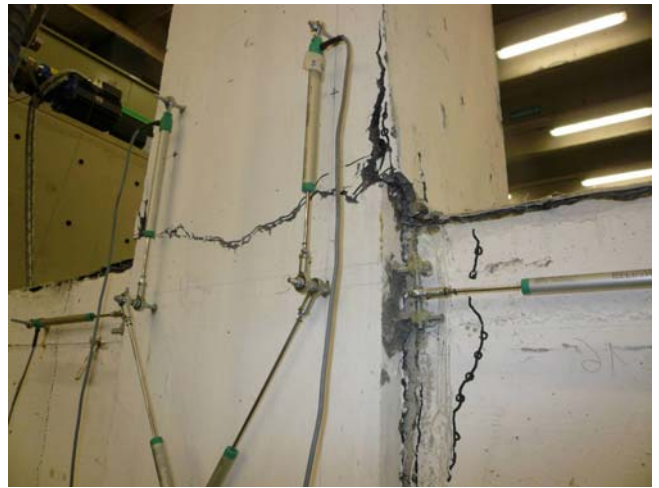
Figure 11. Failure of the column at the top.
